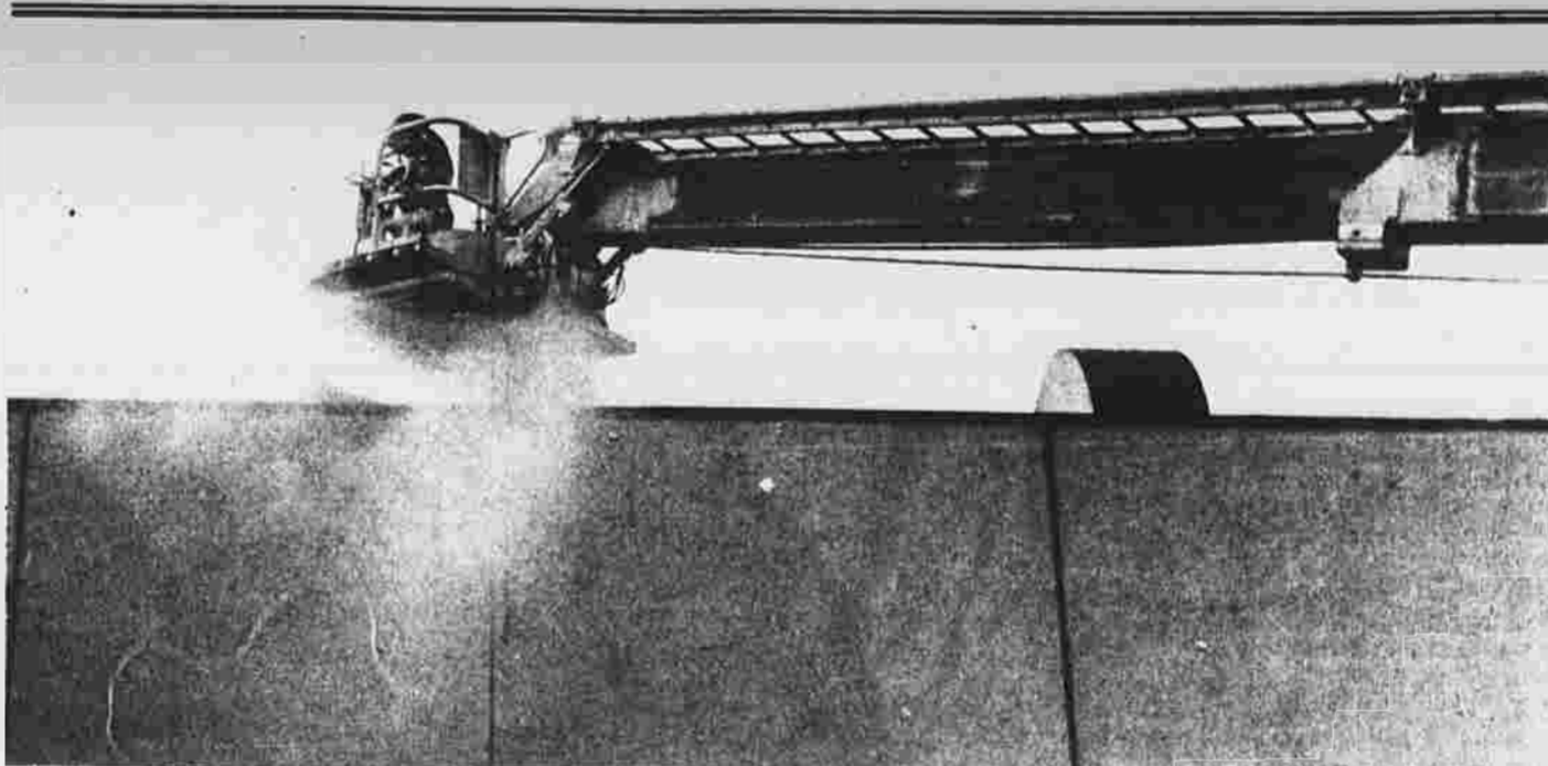
Eighth Utilities District firefighters use their aerial tower Tuesday afternoon to get to the roof of The Donwell Co. on Sheldon Road to battle smoldering ceiling joists they were not able to reach from inside the building.
